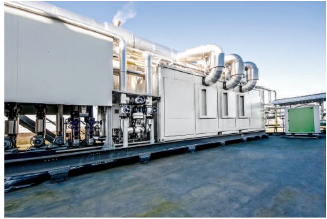
The Capstone C600 system produces heating, cooling and steam for Surgital's new storage warehouse.
